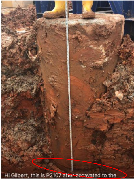
Figure 15. Photo of excavated pile head showing the horizontal crack (Case 4, Site E).
