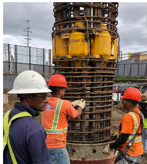
Fig. 2. BDSLTL testing. Installation of steel cage for the pile with cell welded on. Ref. Photos from Universal Tower project.
