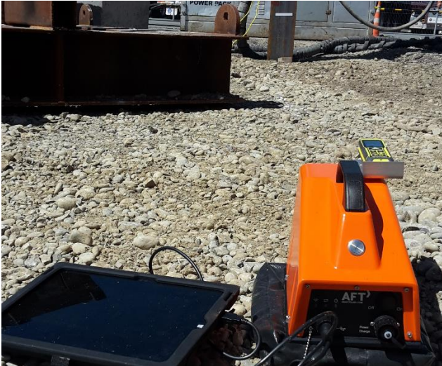
Fig. 3. Example of pile driving monitor set up on site, with reflector sticker on pile.
