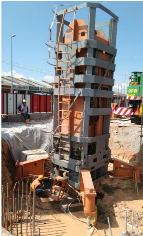
Fig. 4. The field setup of a new drop weight system for HSDLT on drilled shaft.
