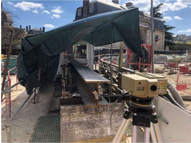
Fig. 6. Testing underway, footprint is the same as the foundation element. The beam is for datum reference only.
