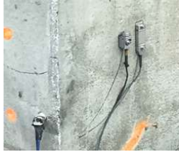
Fig. 2. Typical external gauges installed on concrete piles.
