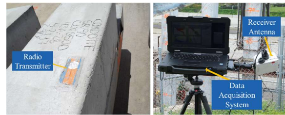
Fig. 4. EDC sensor pack radio transmitter, acquisition system.
