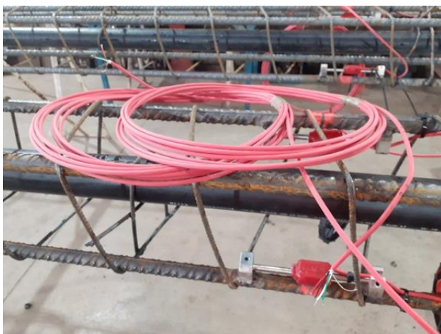
Fig. 2. Vibrating wire extensometer.
