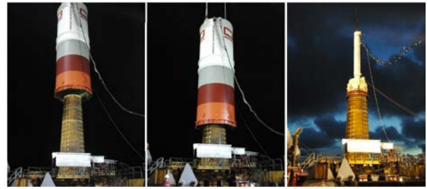
Fig. 10. The installation of a 6.5 m pile with the use of a Noise Mitigation Screen (IHC Offshore Systems) at the German offshore wind farm Riffgat in the North Sea. In the left and middle pictures, the NMS is positioned by the crane around the monopile. In the right picture, the hydraulic hammer is positioned at the head of the pile and the NMS is invisible. Source: Author's personal archive from the Riffgat Offshore Wind Farm (2012).
