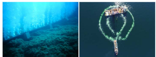
Fig. 7. (Left) Air-bubble cloud released by a perforated pile positioned on the seabed. (Right) Double Big Bubble Curtain (DBBC) deployed around the Giant7 floating piling vessel in the Wikinger OWF, Germany. Source: © Hydrotechnik Lübeck GmbH ( https://www.hydrotechnik-luebeck.de/blog/portfolio-item/0003-borkumwest2-00/ ).
